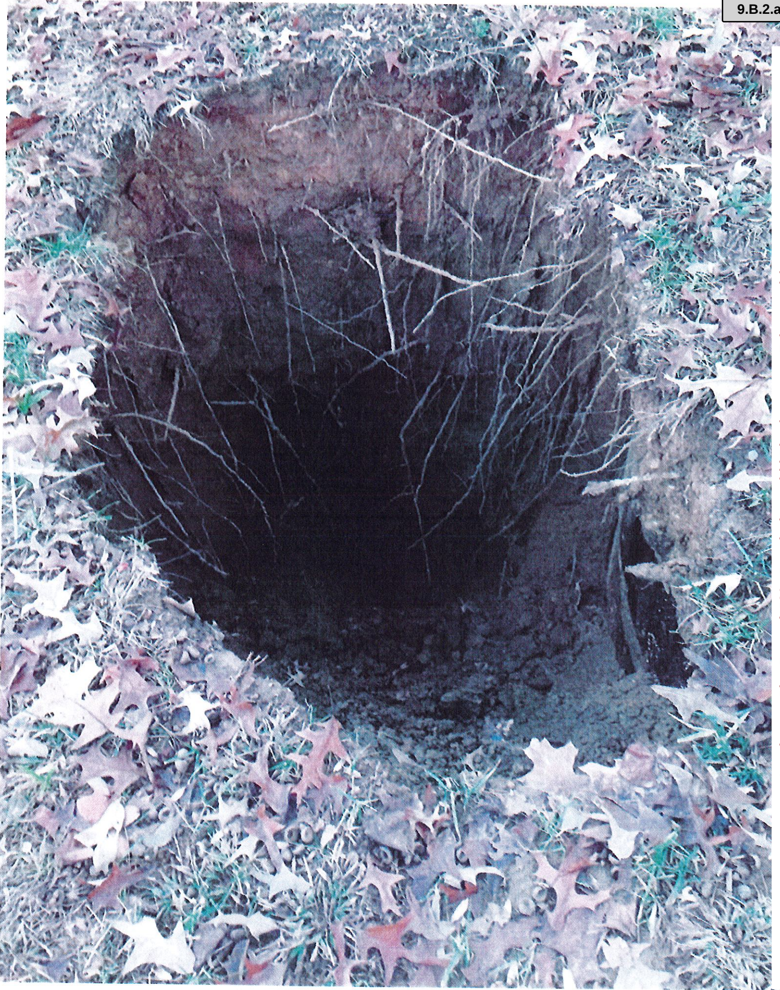
Attachment: Pipe Burst (1536 : Permission to bid Pipe burst near Fairgrounds)
